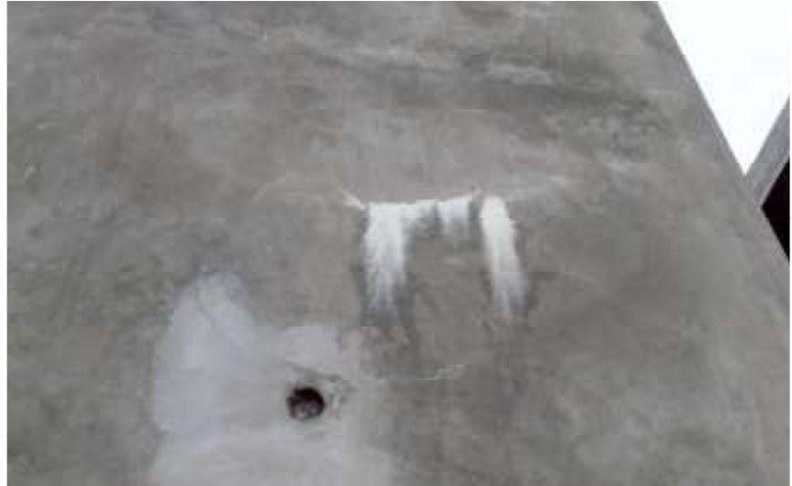
Efflorescence as white deposit and cracking on the complete wall
