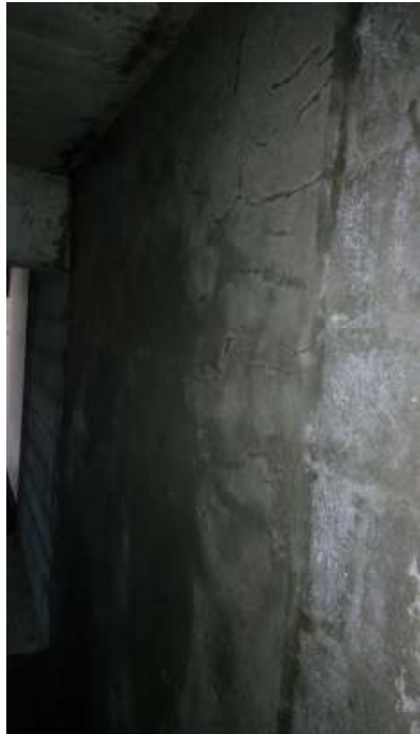
Wall done with CRF, cracked in less than 5 days
