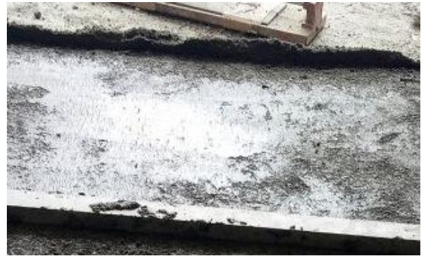
Water-sheen appearing on the surface
